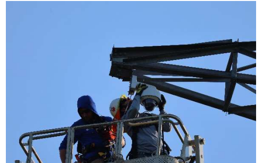
A new Axis 4K PTZ camera is installed on the upper arm of the tower nest. Martin Gaston, Aug. 9, 2025.
